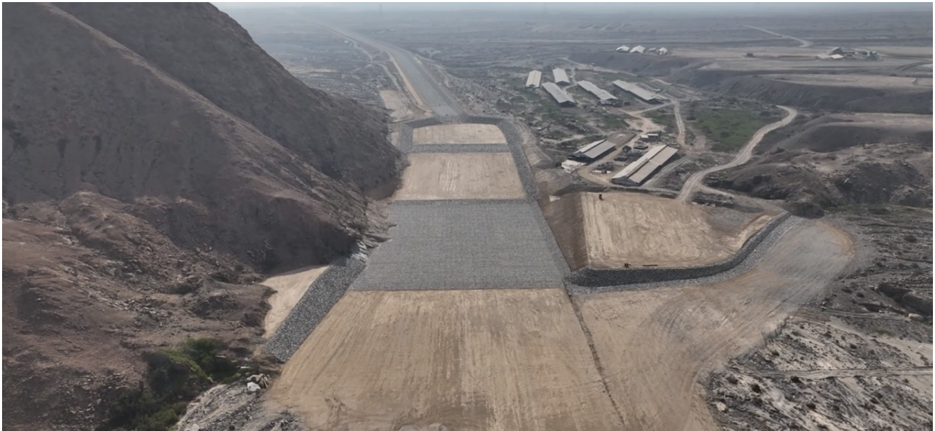
Intake canal structure near poultry farms – all structures were optimized to avoid impact on local industries
