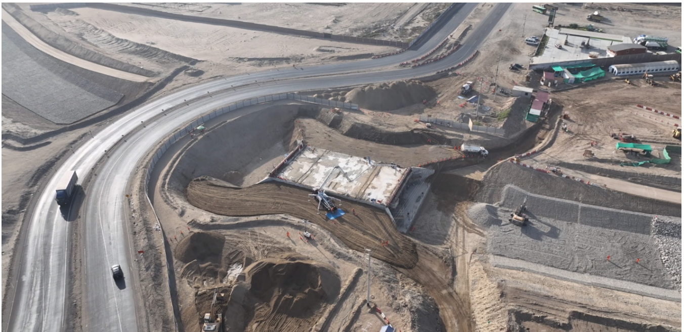
Deviation for construction of the canal crossing of the national highway (Pan-American)
