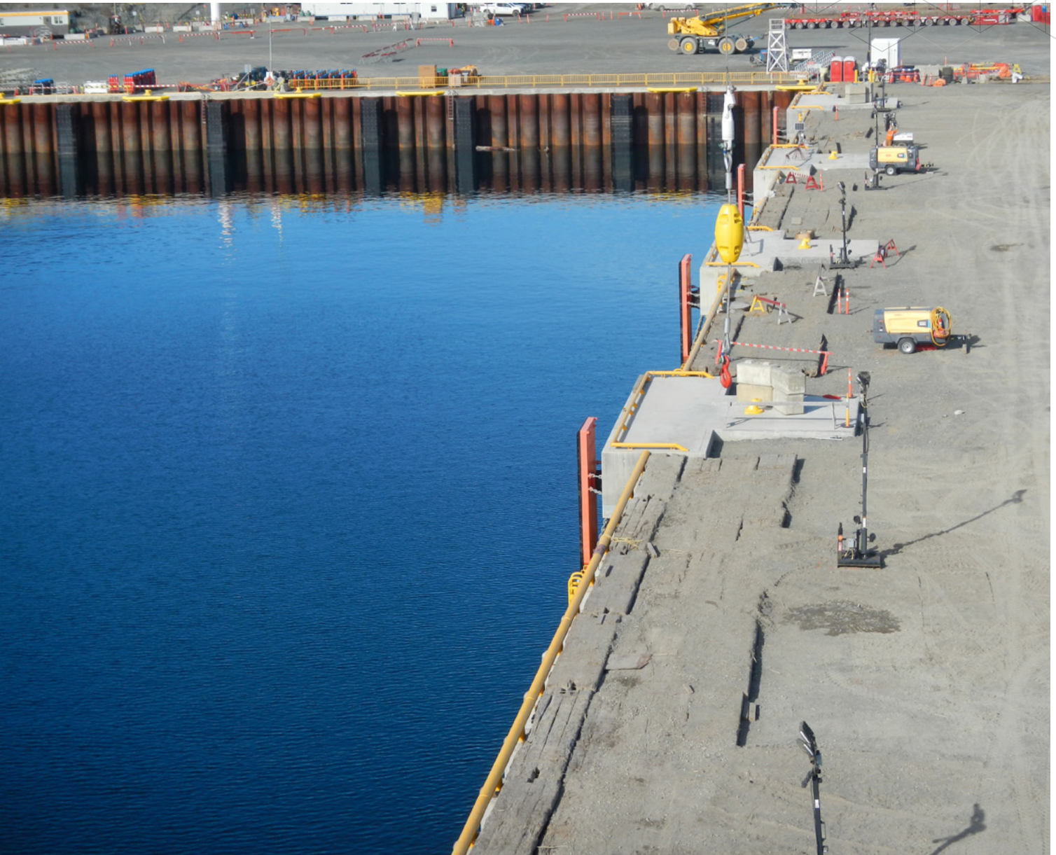
■ MOF North Wall with fender panels post construction (shown as upper bulkhead wall in image)
