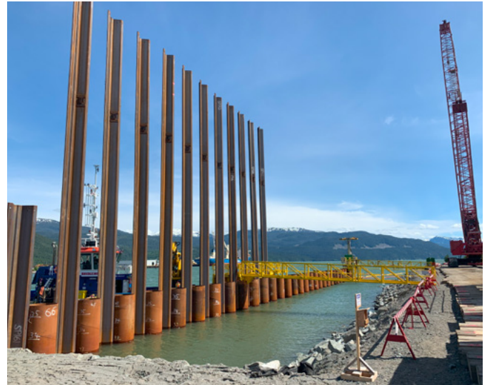
■ Installing infill sheet piles for the combi wall on South end of the West side of MOF
